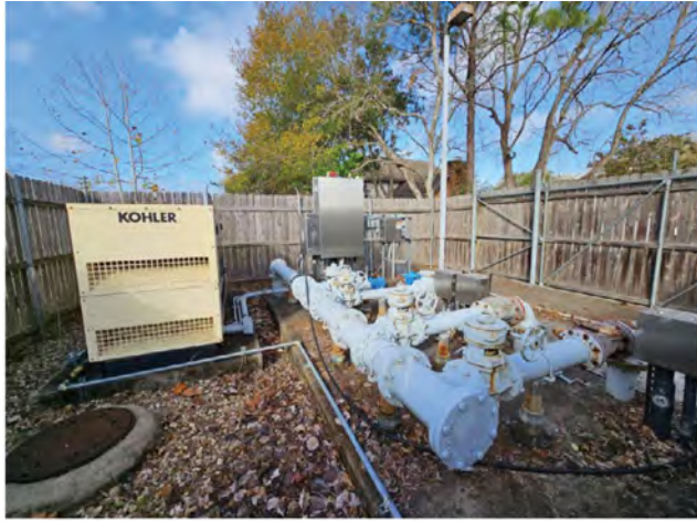
Figure 3 - Lift Station Photograph
